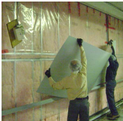
Insulation of R-10 insulation at the inner portion of the dock at Thermoforming Plant 1
