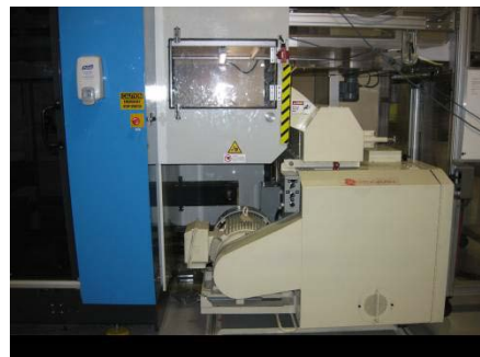
The in-line grinder at Thermoforming Plant 2
