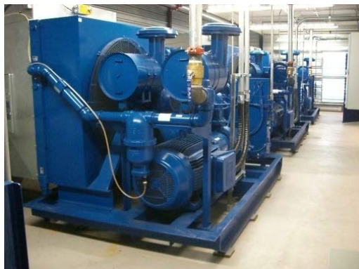
The newly installed compressor at Thermoforming Plant 1
